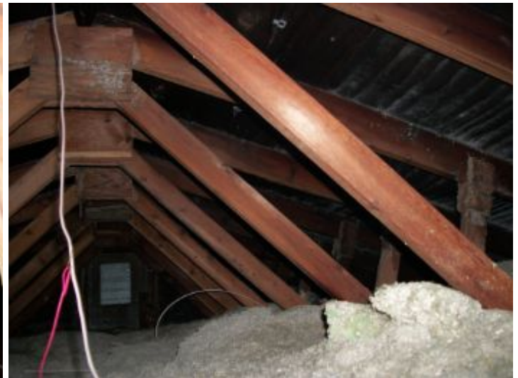
More wet roof sheathing and frost accumulation
