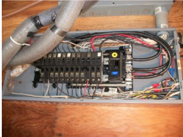
Electrical panel cover removed
