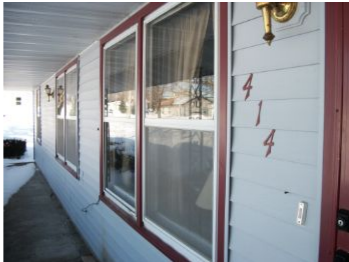
Single pane old windows missing glazing
